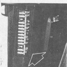
FUSE-BOX lid removed shows simple fuse set-up. Fuses are indexed — legend appears in box-lid.
